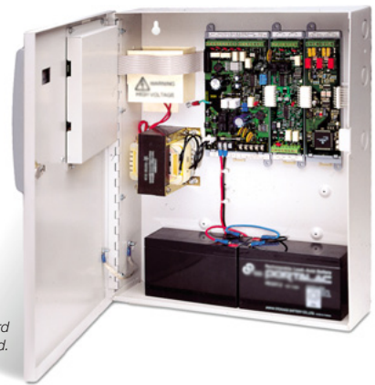
Cabinet with option card and batteries installed.
